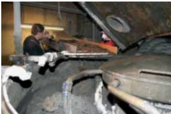
Fig. 4 The steel fibers are added slowly and in a controlled manner; the exact amounts have been weighed and proportioned in advance.
