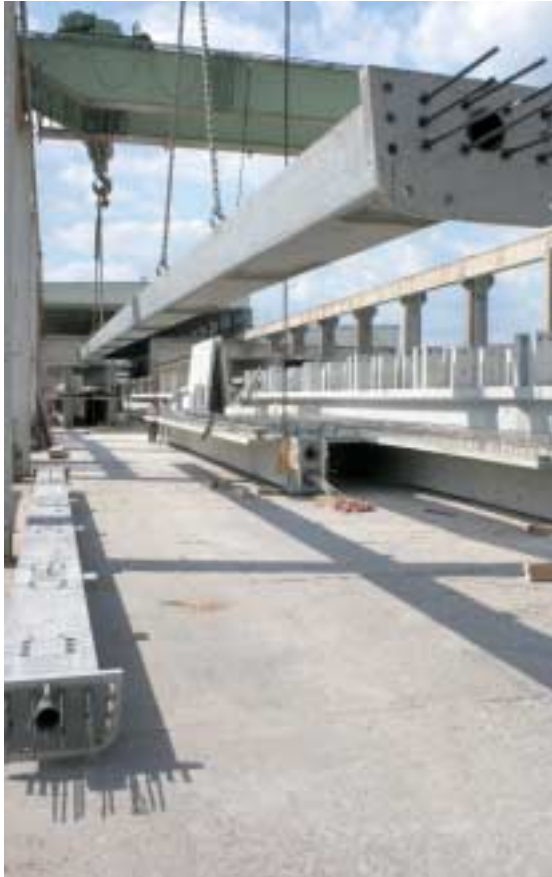
Fig. 12 Already completed upper chords made of UHPC: The upper chord segments are manufactured in lengths of just short of 40 m.
